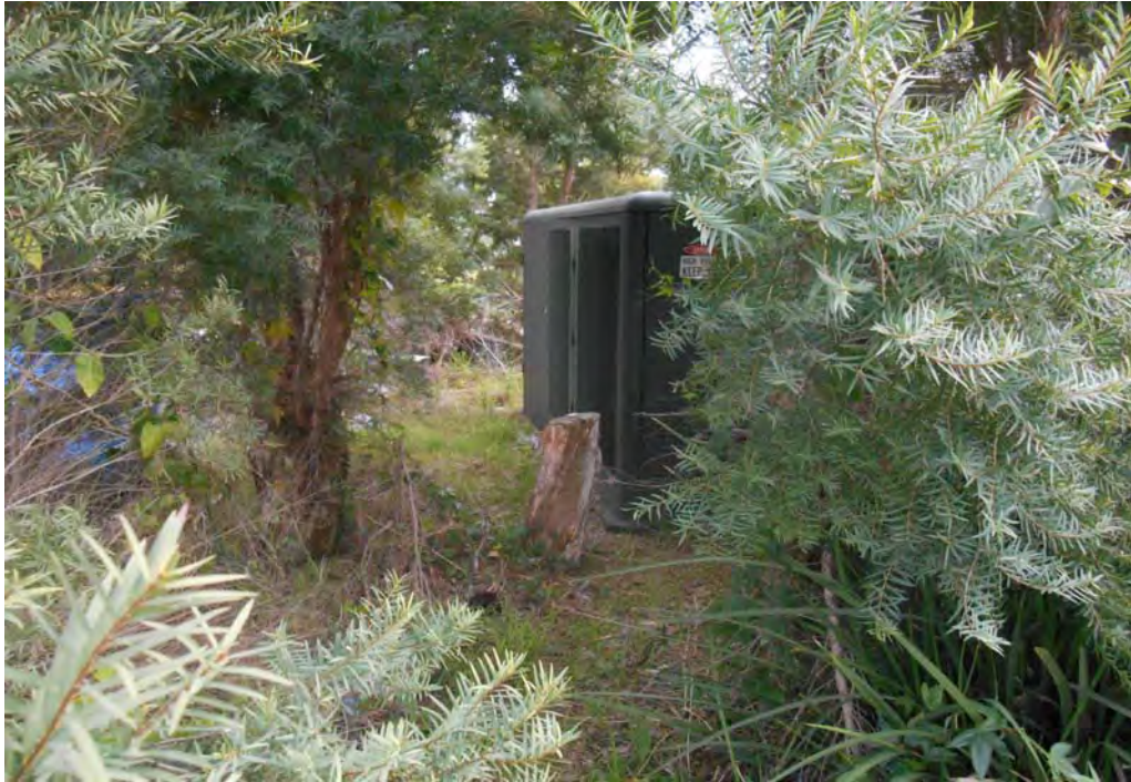
Photograph 1 - Substation at north of site
